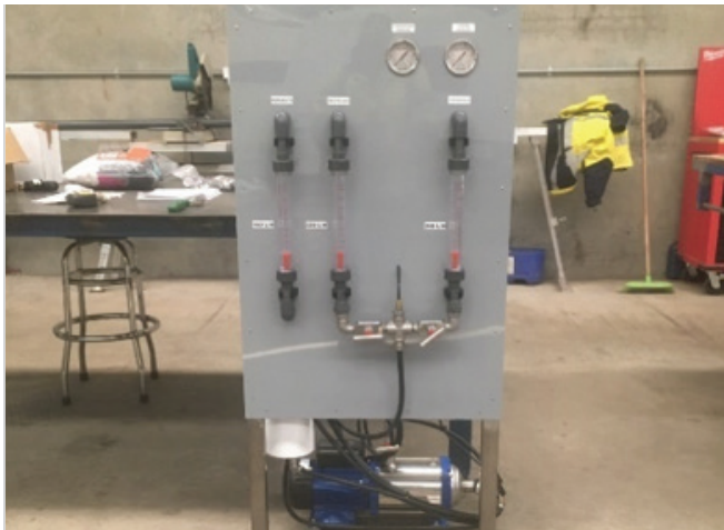
Nano Filtration Pilot Plant.
