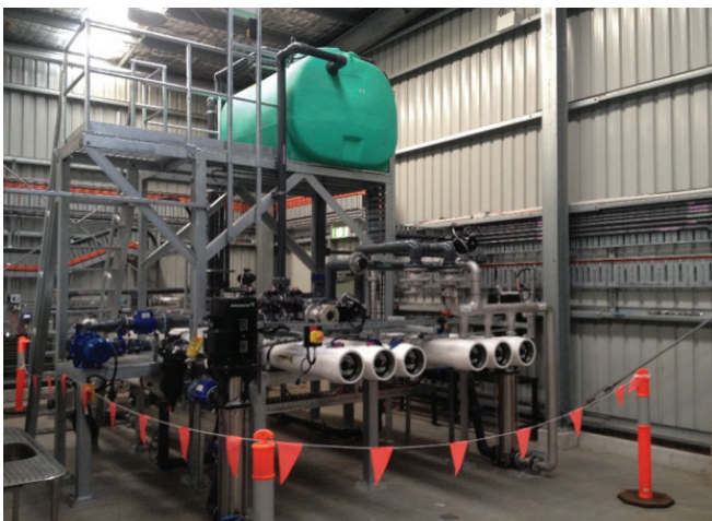
Brackish Water Reverse Osmosis Plant with gravity permeate flush.
