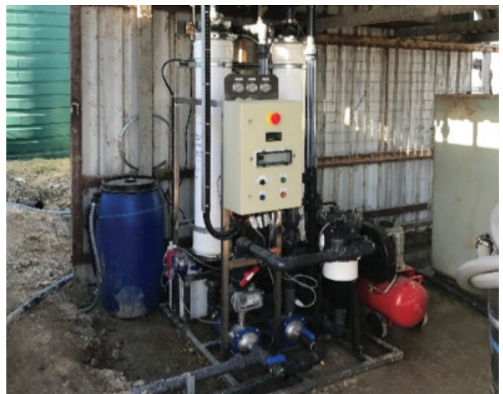
Plant installed onsite.
